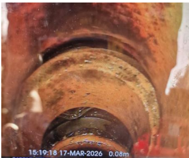
Figure 8: Photos of defects that have been remediated
