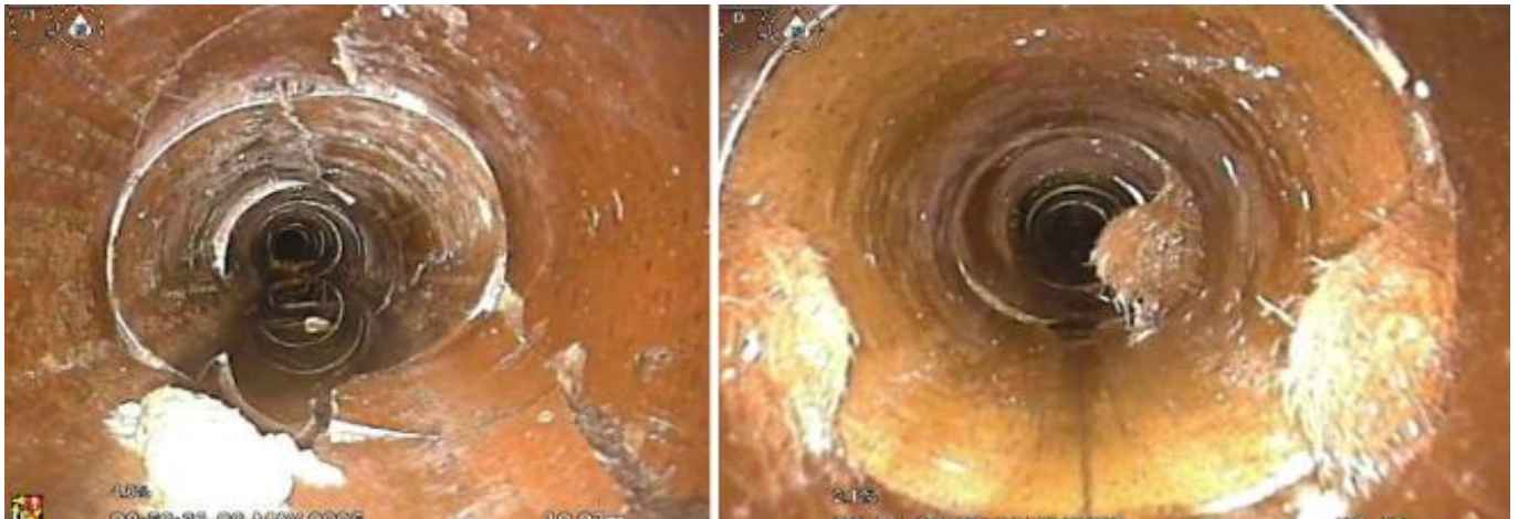
Figure 10: Screenshot of CCTV footage showing multiple severe fractures in sewer before rehabilitation was completed
