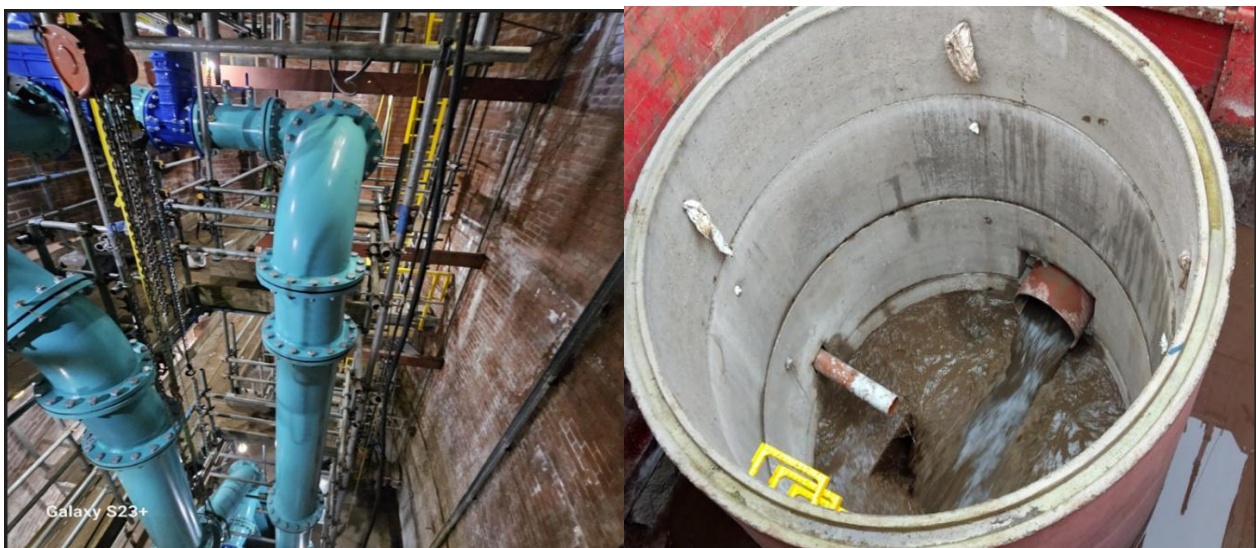
Figure 14: New transfer pumping station and manhole connection to transfer flows from the high-level inlet to low-level inlet
