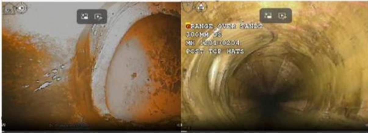
Figure 13: Before and after images within Grange-over-Sands network demonstrating presence of groundwater infiltration (left) and remediation through a lateral connection repair known as a 'top hat' (right).
