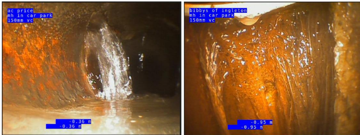
Figure 16: 2022 CCTV surveys identified evidence of groundwater infiltration within Ingleton catchment
