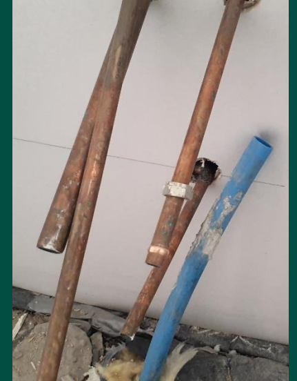
Pipework not ready
