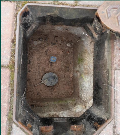
Chamber needs clearing out
