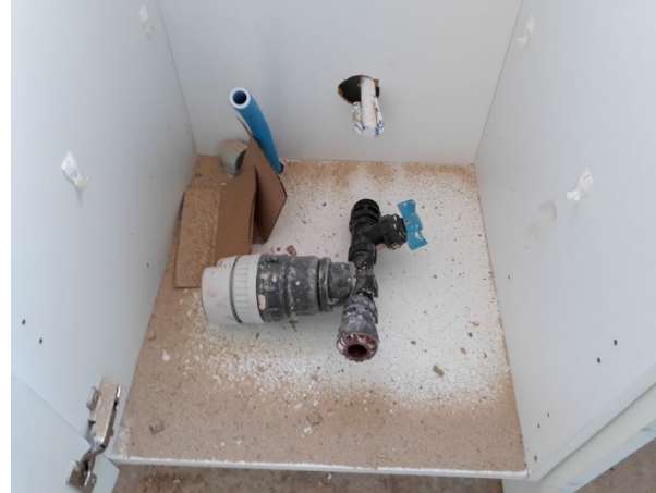
Internal meter install poor practice
